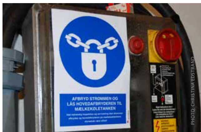
Main switch with warning sign.
